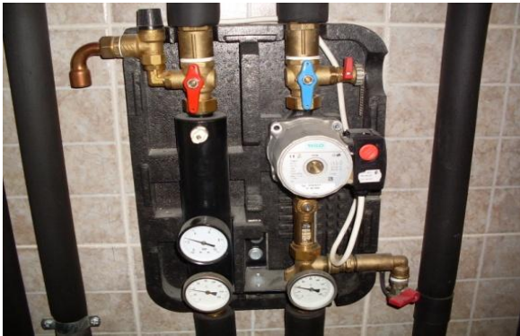
Figure 4.a. Solar station „FV 70 TACOSOL ZR”
