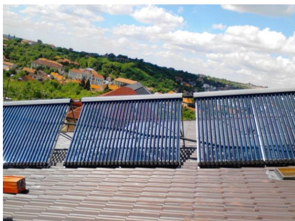
Figure 3.a. Solar collectors Webstech WT-B58-30 with 3x30pc vacuum pipes
