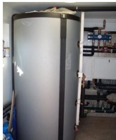
Figure 3.b. Solar reservoir „tank in tank Siss 900/200”
