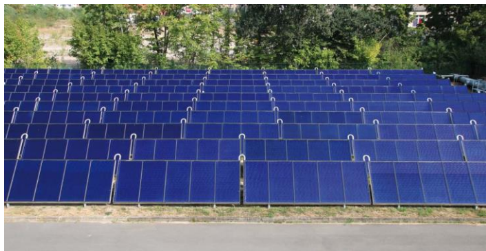
Figure 15: A 0.7 MW th solar thermal system supplies heat to the Berlin district heating network.
