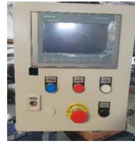
Figure 4. Siemens control panel with a touch display
