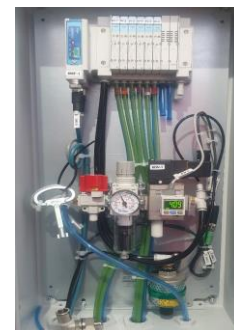
Figure 17. The pneumatic panel
