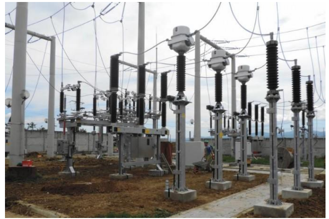
Figure 10. Power Substation from Ștei, Bihor
