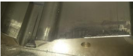
Figure 5. Support worn out.
